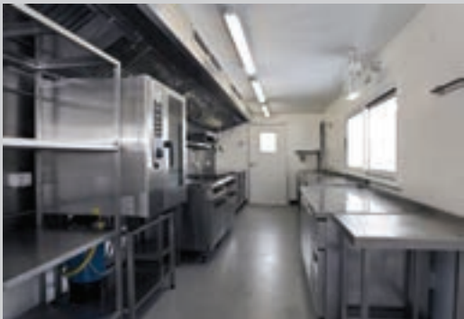
Portable cold rooms and temporary kitchens
